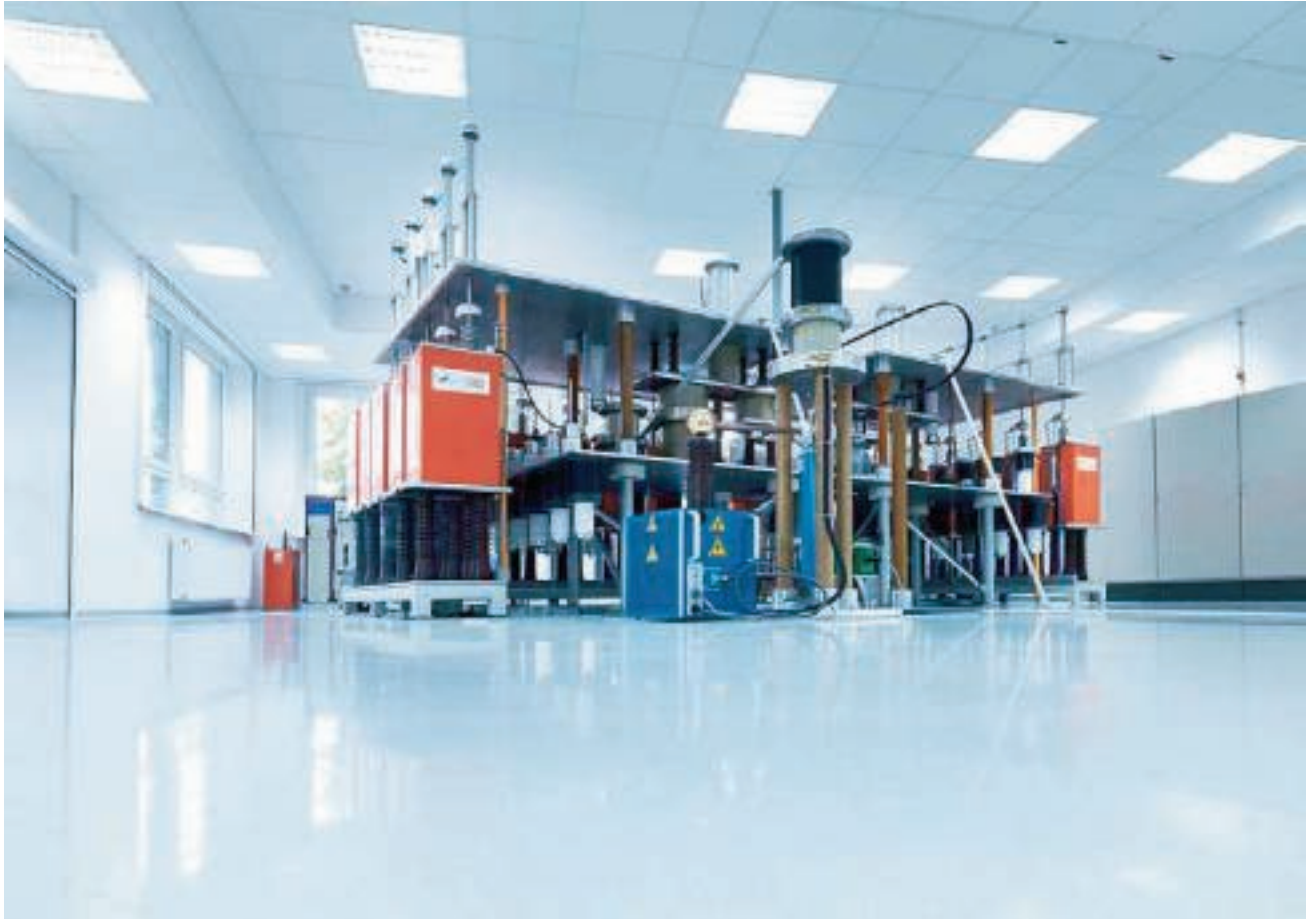
Lightning current test
