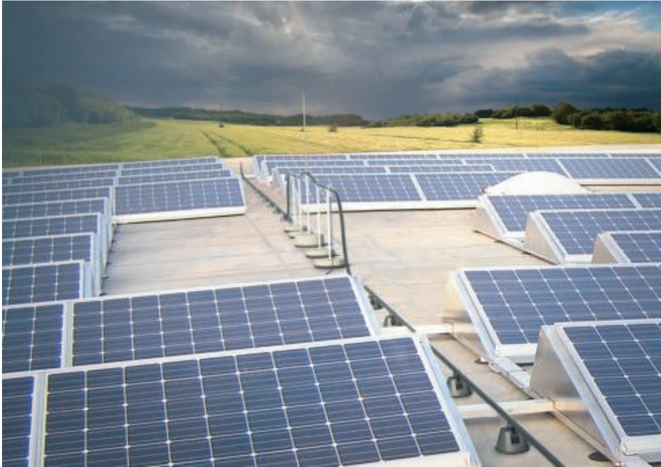
Flat roof with PV system and insulated isCon® cable
