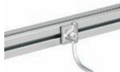
Lightning protection equipotential bonding on the PV mounting system
