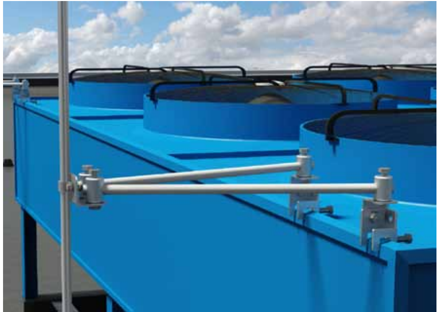
Insulated lightning protection with GfK holder on cooling unit
