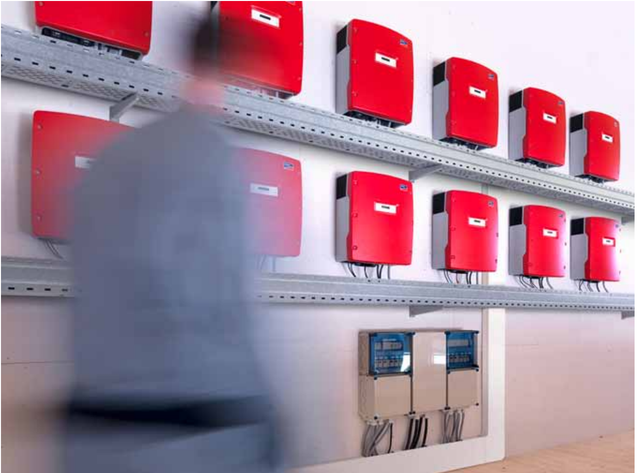
Cable routing with cable support system and plastic wall duct and surge protection
