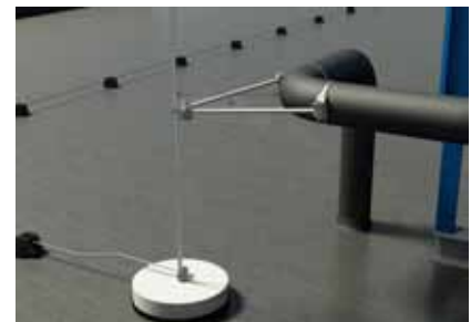
Insulated lightning protection with GfK holder on pipeline
