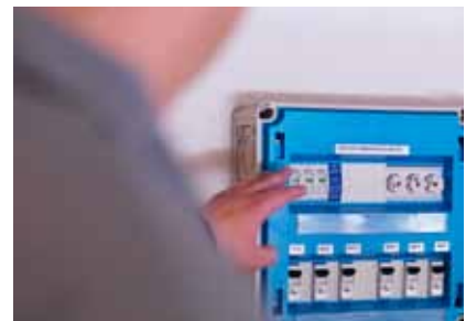
Surge protection on the AC PV distributor
