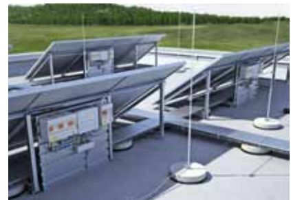
Insulated lightning protection and combination arrester on inverter
