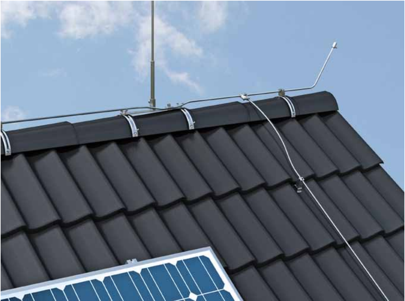
Sloping roof with PV and lightning protection systems
