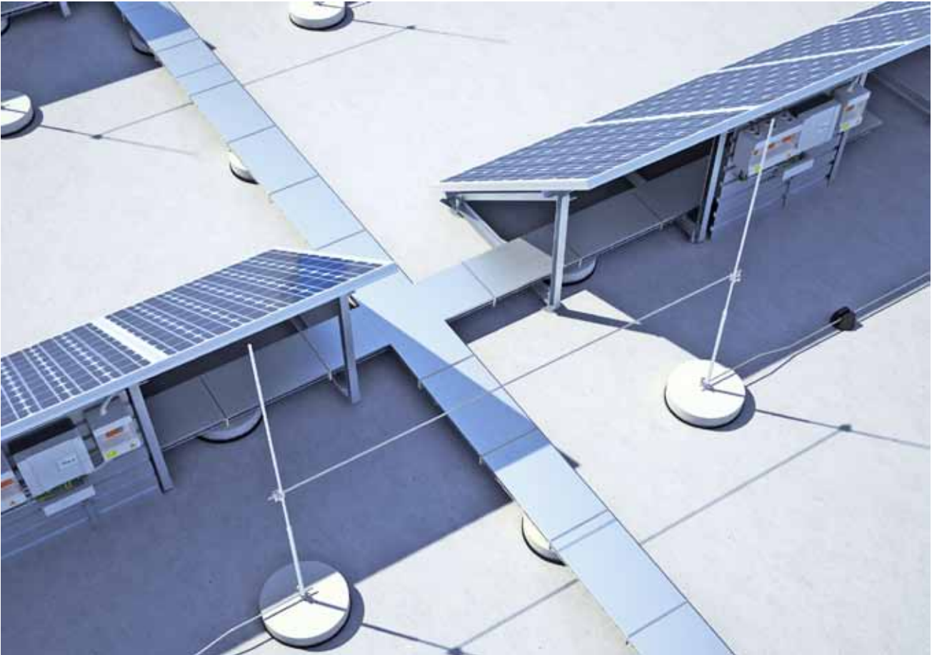
Separation distance ( s ) between the lightning protection system and cable support system
