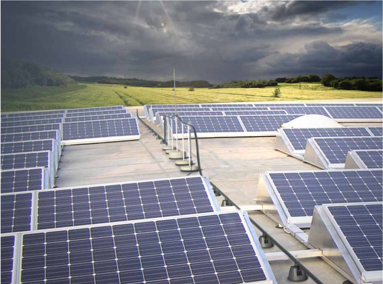
Flat roof with PV system and insulated isCon® cable
