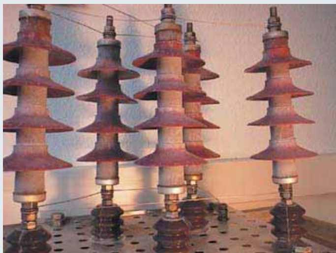
Fig. 1: DEHNmid arrester with considerable salt deposits after a 5000 hours test with cyclically alternating stress including rain, saline fog, temperature fluctuations and UV radiation at a continuous voltage U_C .
