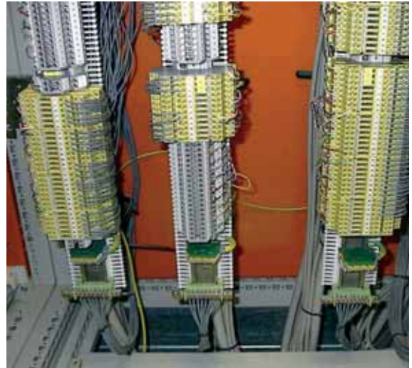
Fig. 9.4.8 DCO ME 24 surge protection device installed into a switchgear cabinet, incoming lines from double bottom
