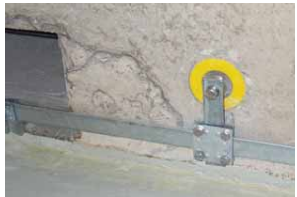
Fig. 7.7.1.1 Ring equipotential bonding and fixed earthing point for connection of metal installations
