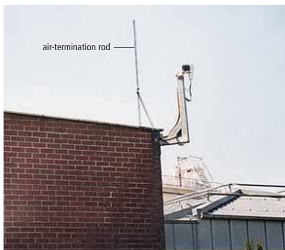
Fig. 9.7.2 Camera for video surveillance in the protective area of the air-termination rod
