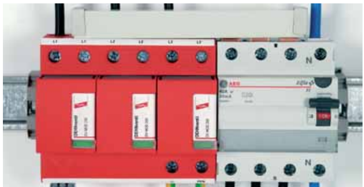
Fig. 8.1.6.11 V-shape series connection of the DEHNventil M TNC combined lightning current and surge protective device by means of a busbar
