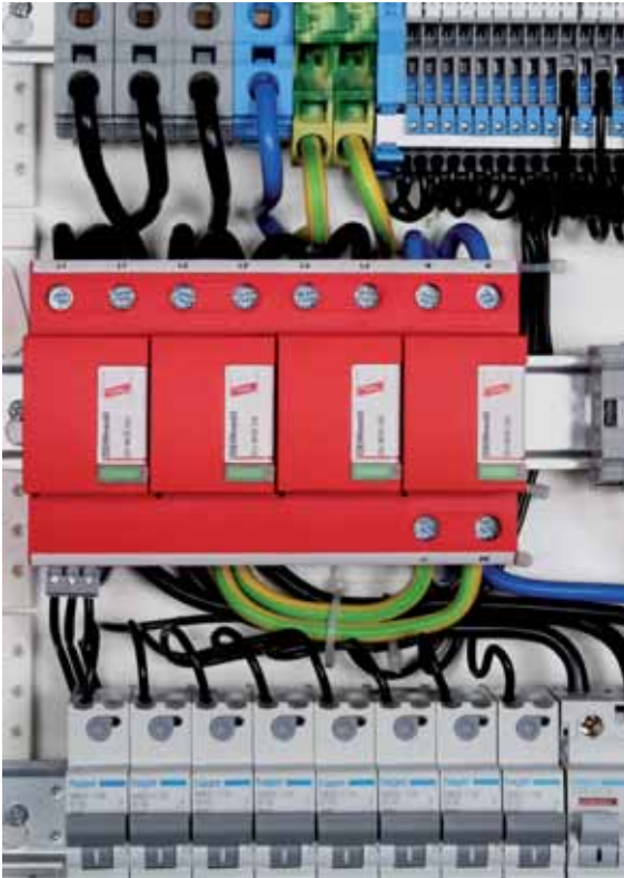
Fig. 9.4.6 DEHNventil installed into a switchgear cabinet for protection of the power supply system
