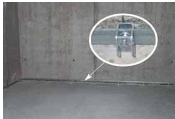
Fig. 7.4.2 Ring equipotential bonding bar in a computer facility
