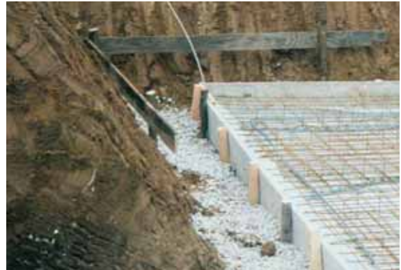
Fig. 5.5.2.4 Foundation earth electrode in use
