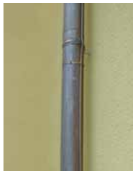
Fig. 5.2.2.2.4 Down conductor installed along a downpipe
