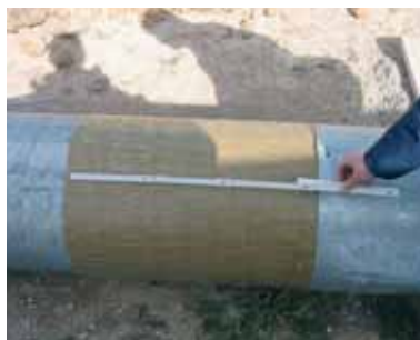
Fig. 5.1.8.8 Additional protection in the transition area by anticorrosive band for underground application
