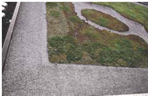
Fig. 7.3.7b Use of galvanised construction steel mats for shielding, e.g. in case of planted roofs
