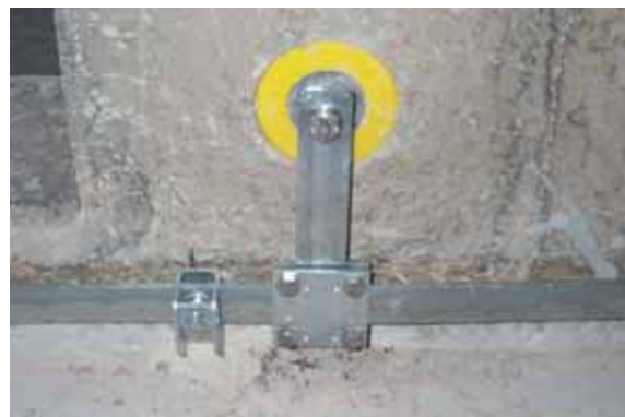
Fig. 7.4.3 Connection of the ring equipotential bonding bar with the equipotential bonding network via fixed earthing point
