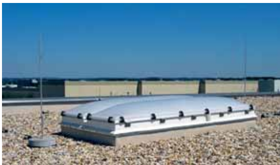
Fig. 5.1.1.17 Protection of small-sized installations on roofs against direct lightning strikes by means of air-termination rods
