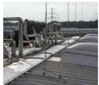
Fig. 5.1.4.7 Air-termination rod for a dome-light on a roof with round standing seam
