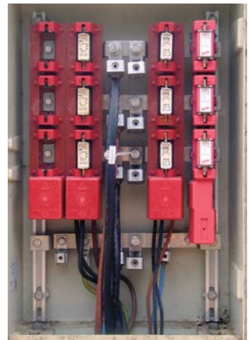
Fig. 8.1.6.6 Surge protective device Type 2 V NH for use in NH fuse bases
