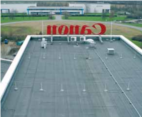
Fig. 5.1.8.10 Installed air-termination system Ref.: Blitzschutz Wettingfeld , Krefeld. Germany
