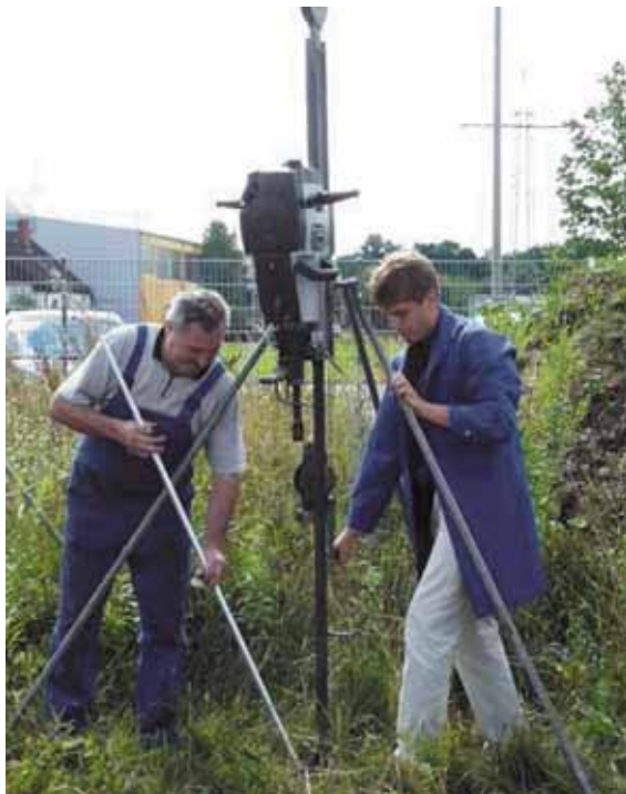
Fig. 5.5.4.2 Driving the earth rod in with a work scaffolding and a vibrating hammer
