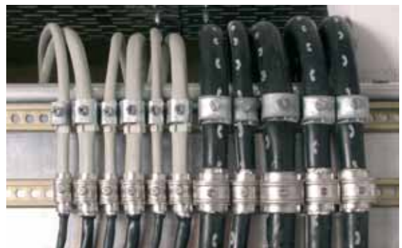
Fig. 6.3.3 SAK shield connection system capable of carrying lightning currents
