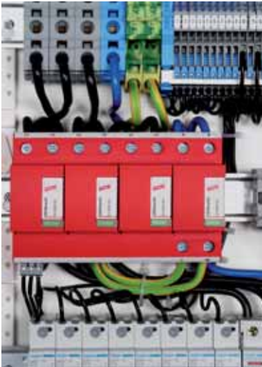
Fig. 9.15.4 DEHNventil DV TT 255 in a switchgear cabinet for protection of the power supply system
