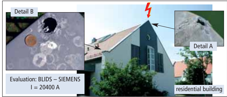
Fig. 5.1.4.2 Example of damage: Metal plate cover
